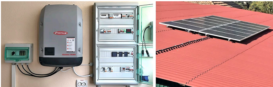
Fig. 5.5 Grid inverter, DC and AC switchgear, and solar panel array installed at the demonstration grid-connected solar power plant
